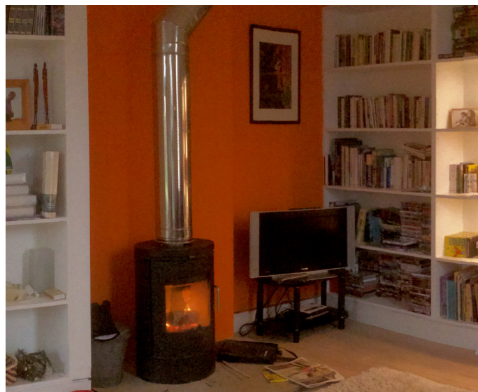
A wood stove can be delightful but there are risks to health from a range of potential gas leaks. This stove has a separate combustion air supply which connects in beneath direct from outside and is 'room sealed' which reduces the risks somewhat.
