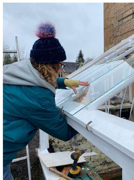
Images: Top: Douglas Fir post & beam frame in Glenrothes for Thomson Timber; K Cassels Bottom: Restoration of Victorian glasshouse in Glasgow; K Cassels
