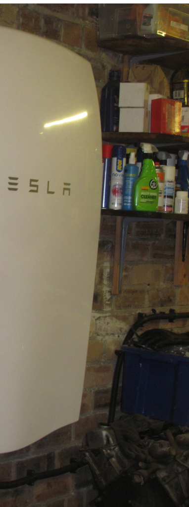
10kW Lithium-ion battery
