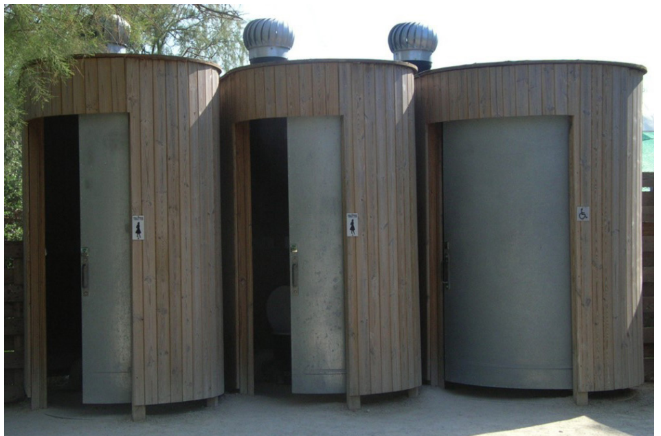
Above: Dry toilet units at a wildlife park in southern France where conventional sewage treatment was deemed to be too damaging to the local waterways.
