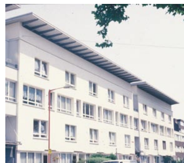
This aesthetic prohibits DfD through use of continuous hard render. Source: F. Stevenson
