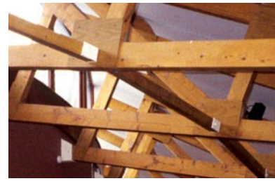
Poorly detailed connectors can prevent effective re-use of timber. Source: F. Stevenson
